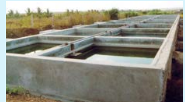
Sludge drying beds
